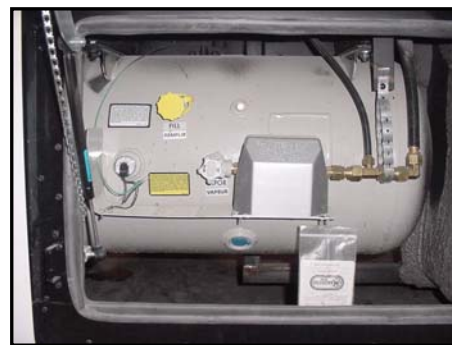
Figure 2-3. Liquid Propane Tank
