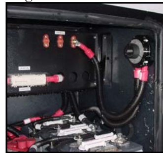
Figure 7-7. House Battery Disconnect Switch (right side)
