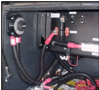
Figure 7-6. Engine Battery Disconnect Switch (left side)
