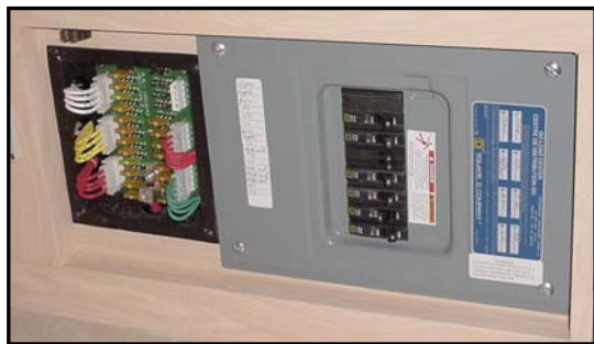
Figure 7-1. Circuit Breaker Box
