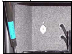
Figure 4-15. Cable & Telephone Jack
