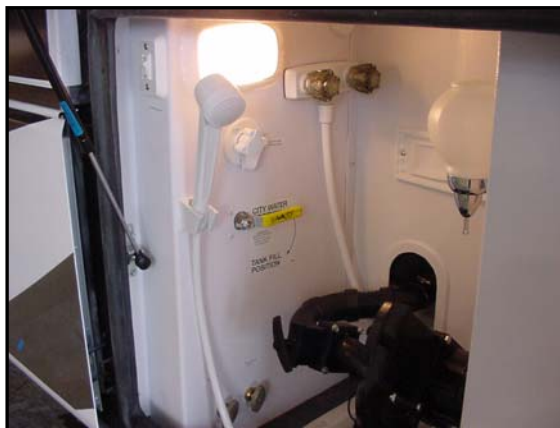
Figure 11-12. Exterior Shower and Exterior Light
