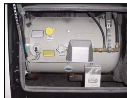
Figure 3-4. Liquid Propane Tank
