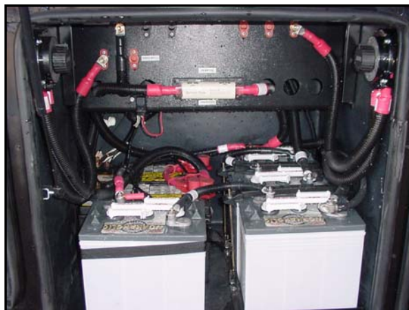
Figure 7-5. 12 VDC Battery System
