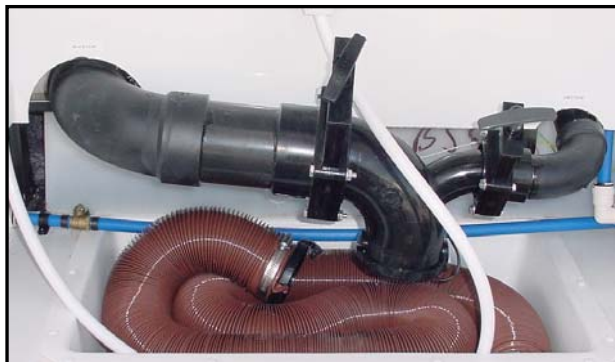
Figure 11-11. Sanitation Coupling, Valve, and Hose
