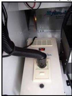
Figure 14-12. Vacuum Cleaner System
