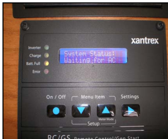
Figure 7-13. Inverter Control Panel
