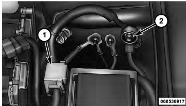
Remote Battery Posts
